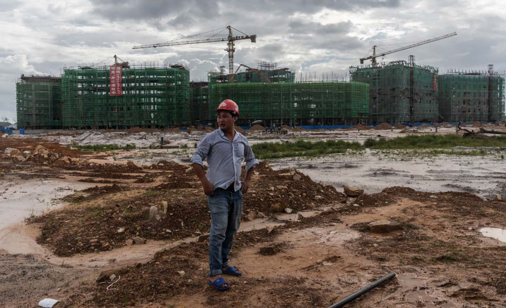
A worker stands on the site of a Chinese construction project in Dara Sakor on August 8, 2019. In 2008, a Chinese state-controlled company secured a ninety-nine-year lease on the area, which includes 20 percent of Cambodia's coastline. (Photo by Adam Dean/New York Times)
