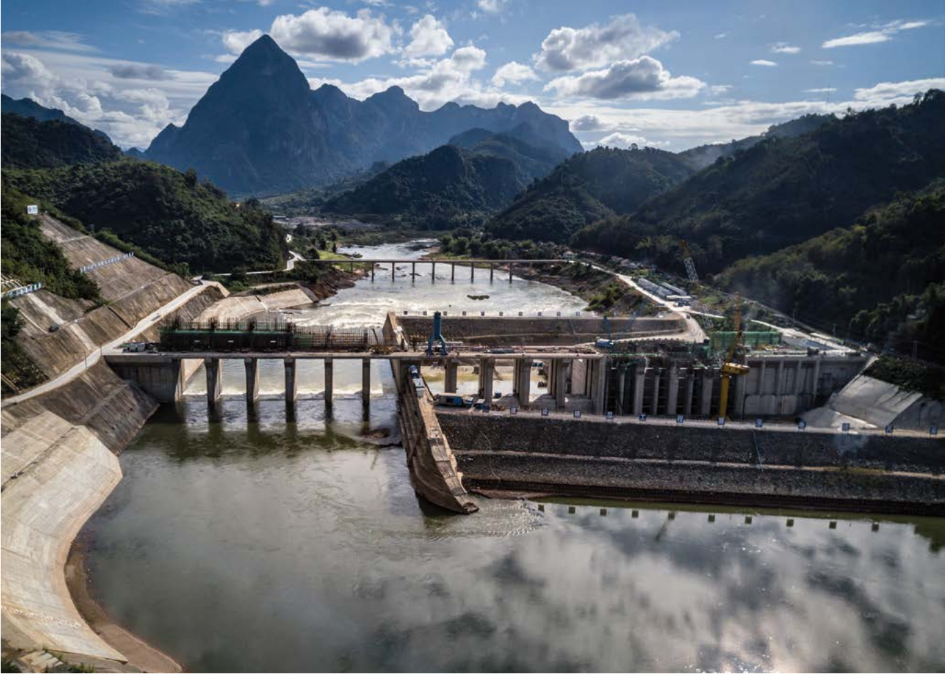
The Nam Ou 1 Dam on the Mekong River in Luang Prabang Province, in northern Laos, under construction on December 10, 2018. It was built by China's largest hydropower company. (Photo by Sergey Ponomarev/New York Times)
