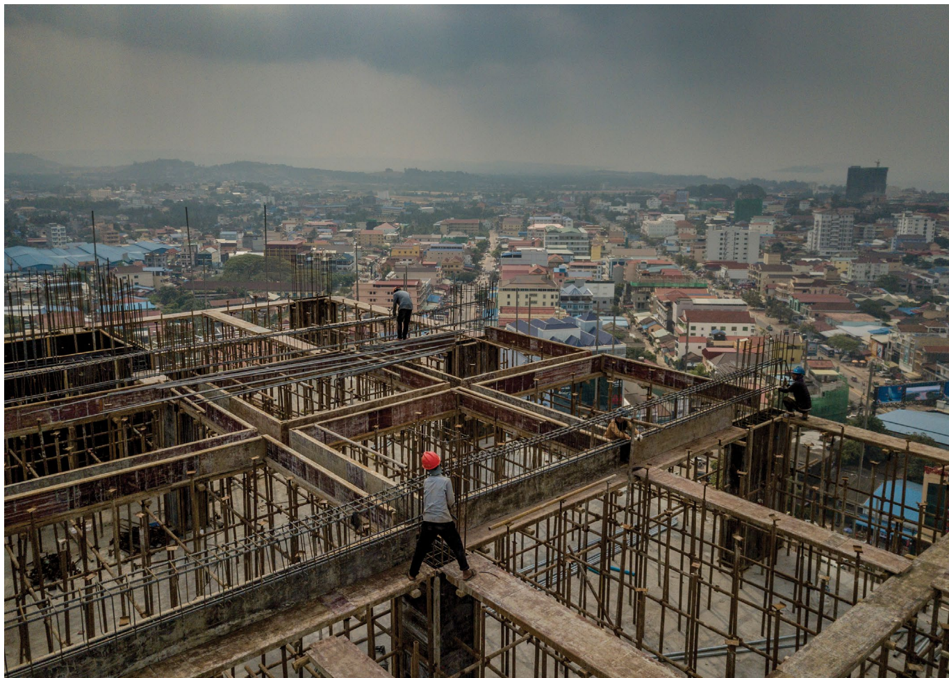
Construction workers work on a Chinese-financed casino, condominium, and hotel development on the seafont in Sihanoukville, Cambodia in February 2018. (Photo by Adam Dean/New York Times)
